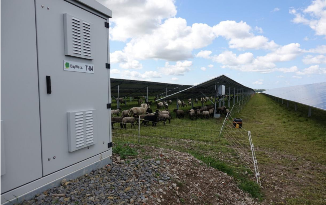
Plate 3: Typical transformer on a solar farm site
