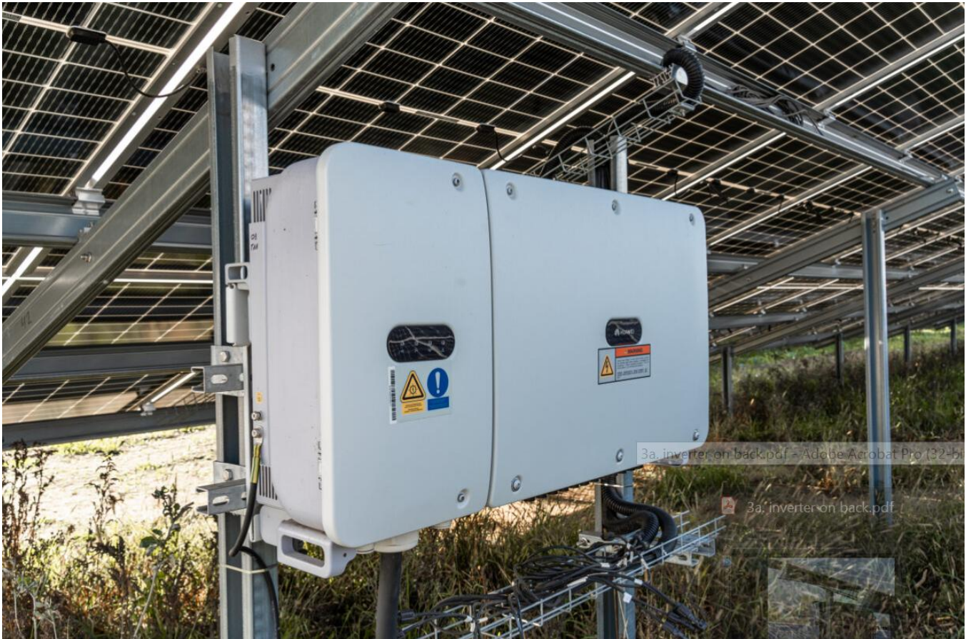
Plate 2: Detailed view of typical mounting structures and string inverter
